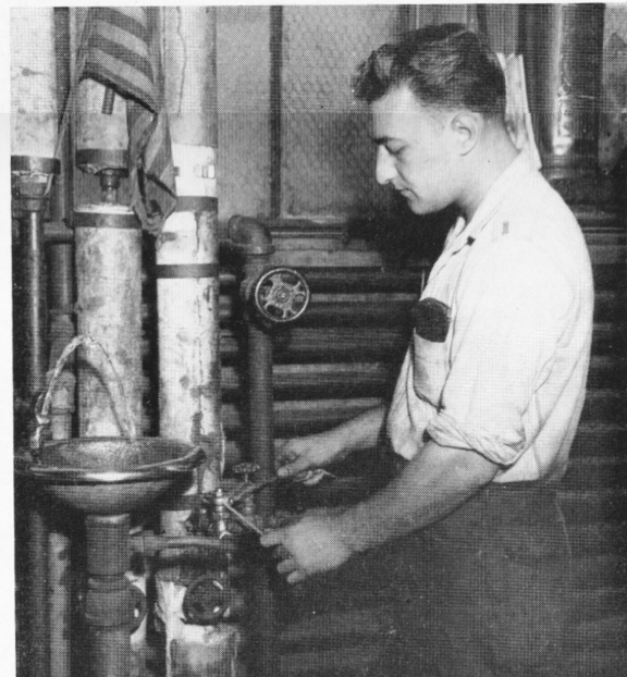
Here is a reason why the cooling system has to race at top capacity. Jim Luttazi, Pipe Shop, shows how some employees waste water: by tying fountain handles in an effort to run cool water colder. The result: wasted energy and warmer water.
